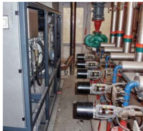
Cogeneration unit with Baelz hydro ejectors
