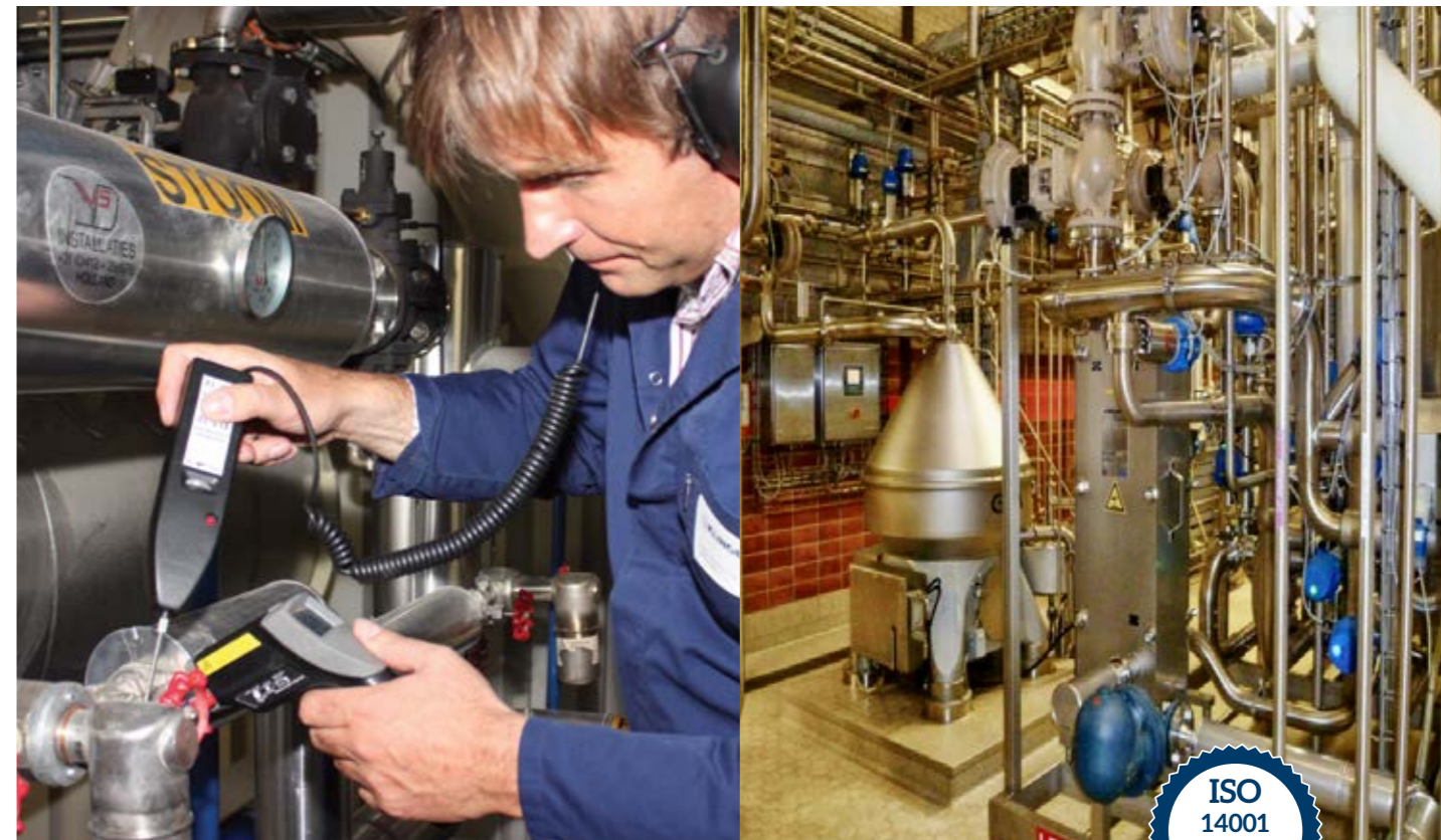
Steam trap survey in progress by a KLINGER engineer
