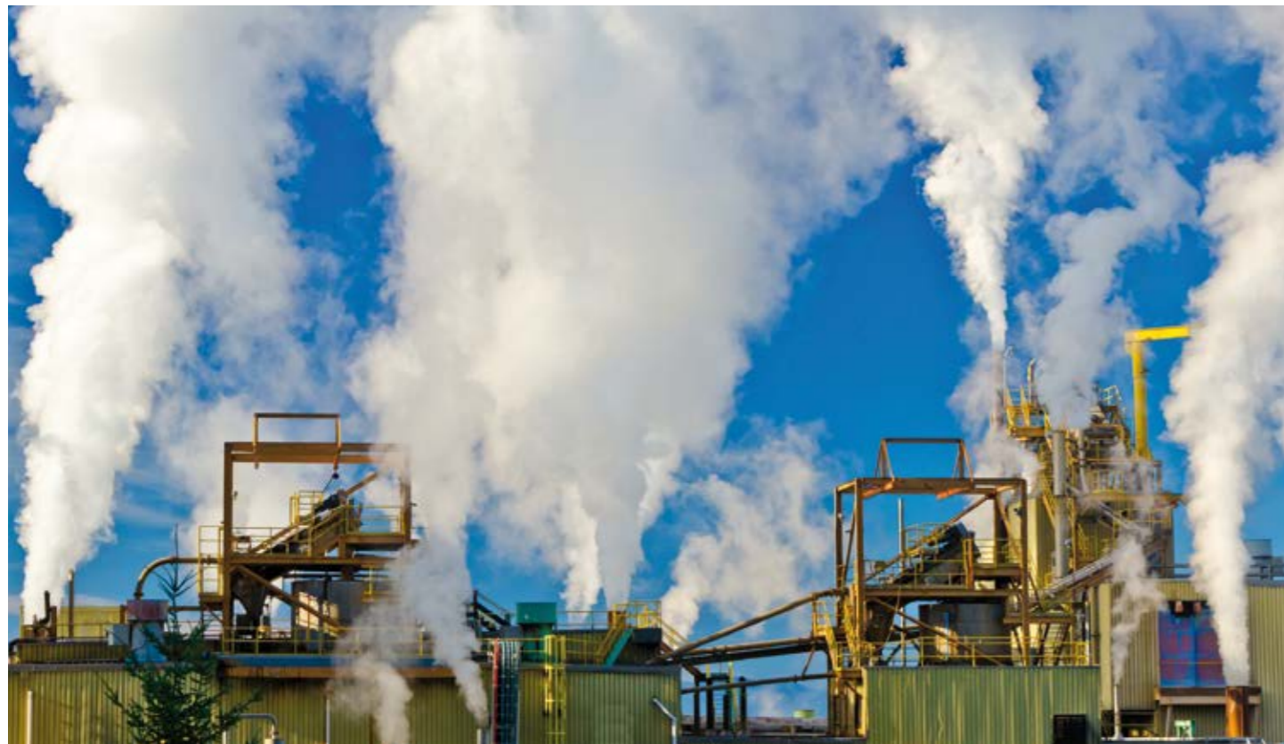
Visible steam losses and the question is: "Where are the leaks"?
