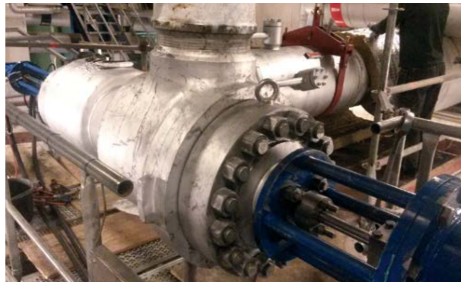
The combined safety shut-off and steam conversion control valve welded in and ready for insulation
